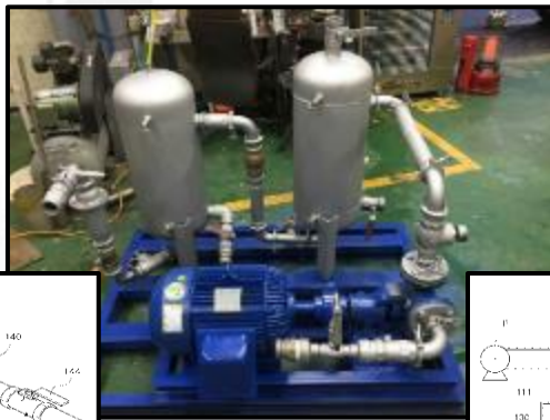
MB generator + Chemical feeder
