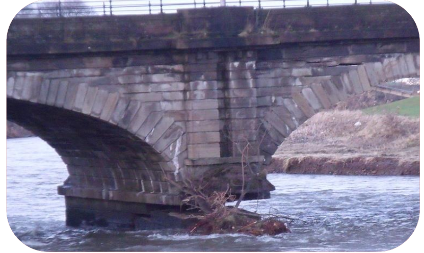
NO PRACTICABLE SERVICE. Calva bridge (2009)
