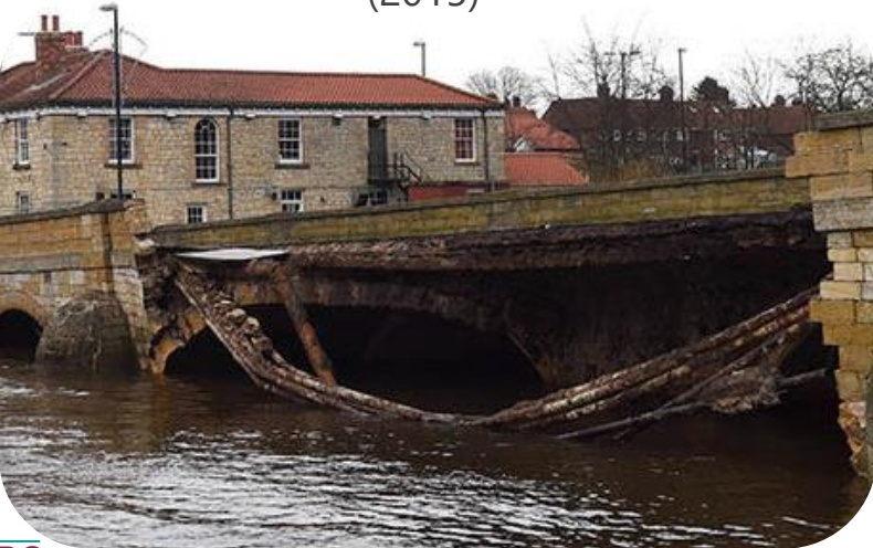
COLLAPSE. Tadcaster bridge (2015)
